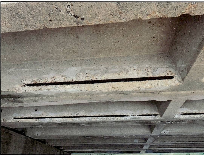
Span 4, units 5 and 6 have widespread exposed rebar. Unit 6, left leg: has lost adhesion at midspan for 2ft.
