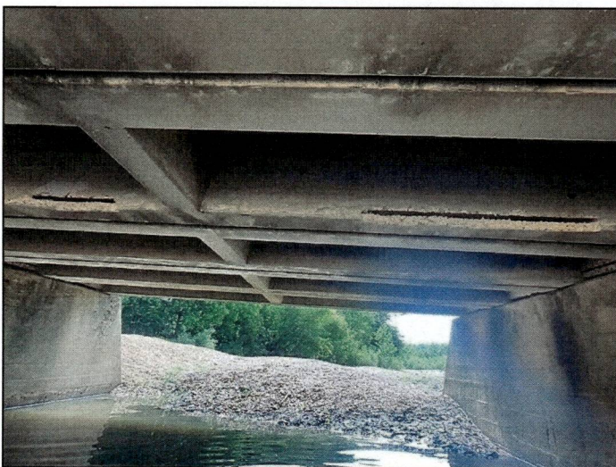
Span 10, unit 3, right leg: has exposed rebar at the 1/4 and midspan points.
