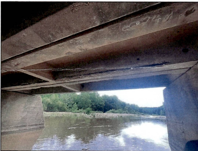
Span 3, unit 5, right leg: has spalling with rebar exposure beginning 1' ahead of bent 2. 7' of the rebar has lost adhesion to the surrounding concrete.
