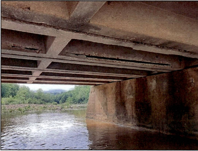
Span 5, unit 2, right leg: has widespread rebar exposure. At the 1/4 point, the rebar has lost adhesion for 4ft.
