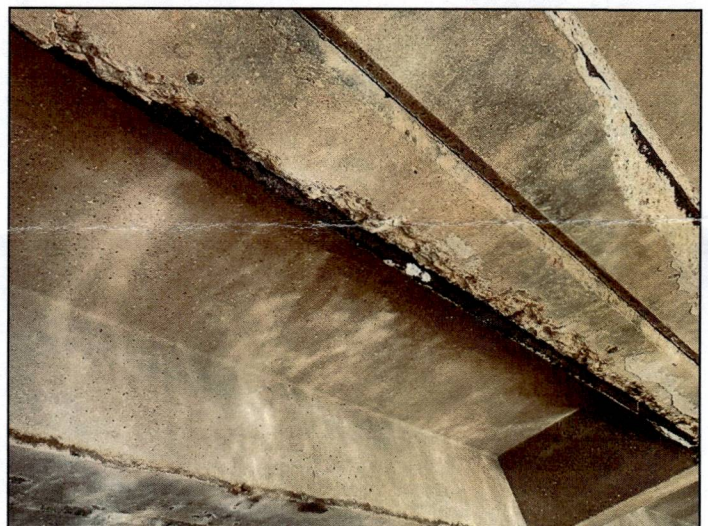
Span 3, unit 5, right leg: has spalling with rebar exposure beginning 1' ahead of bent 2. 7' of the rebar has lost adhesion to the surrounding concrete.
