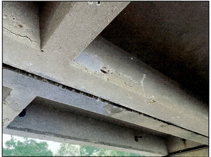
Typical minor exposed rebar.
