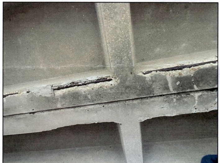
Span 3, unit 1, right leg, midspan: has exposed rebar. The rebar has lost adhesion for 1'.
