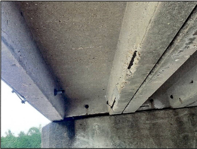
Span 2, bent 2, unit 1: has typical rebar exposure.
