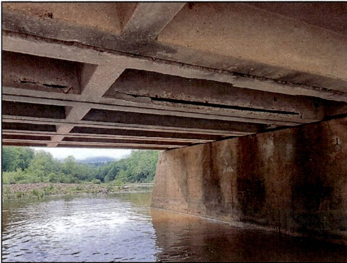
Span 5, unit 2, right leg: has widespread rebar exposure. At the 1/4 point, the rebar has lost adhesion for 4ft.
