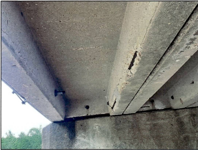
Span 2, bent 2, unit 1: has typical rebar exposure.
