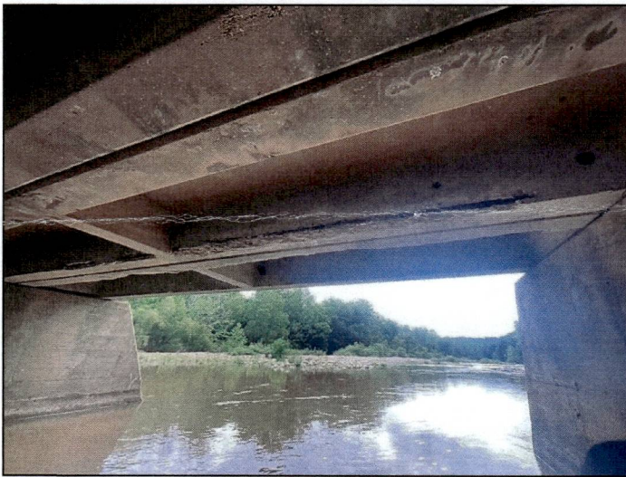
Span 3, unit 5, right leg: has spalling with rebar exposure beginning 1' ahead of bent 2. 7' of the rebar has lost adhesion to the surrounding concrete.
