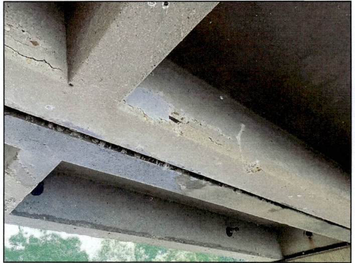
Typical minor exposed rebar.
