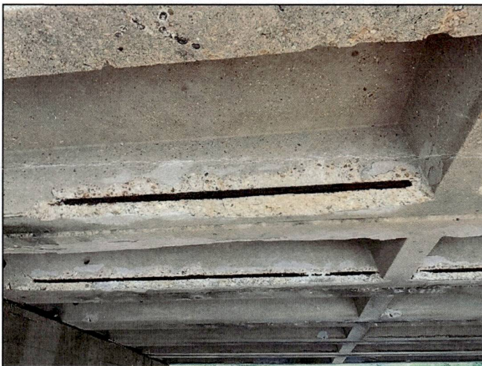
Span 4, units 5 and 6 have widespread exposed rebar. Unit 6, left leg: has lost adhesion at midspan for 2ft.
