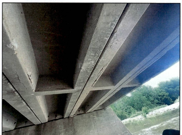
Span 2, units 4, 5, and 6: have spalling with rebar exposed at midspan.
