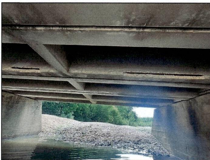
Span 10, unit 3, right leg: has exposed rebar at the 1/4 and midspan points.
