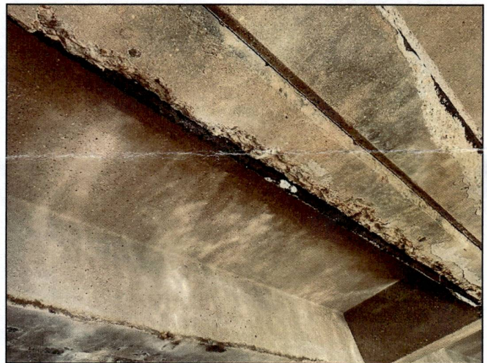
Span 3, unit 5, right leg: has spalling with rebar exposure beginning 1' ahead of bent 2. 7' of the rebar has lost adhesion to the surrounding concrete.
